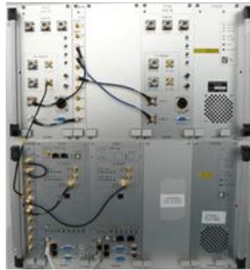
base station (eNodeB)
