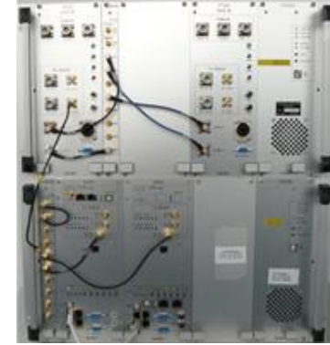
base station (eNodeB)
